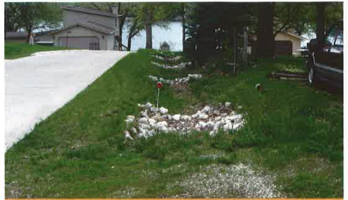
A newly completed bioswale with rock checks in a road ditch above East Okoboji Lake reduces runoff and sediment that used to be delivered to the lake with each runoff event. Rock checks help hold and infiltrate stormwater.
