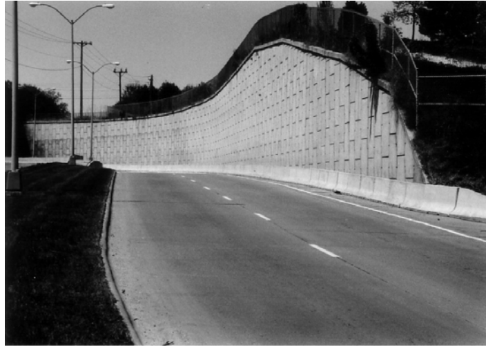
Figure 3.25. Retaining Wall (Source: Department of Civil, Construction, and Environmental Engineering, Iowa State University)
