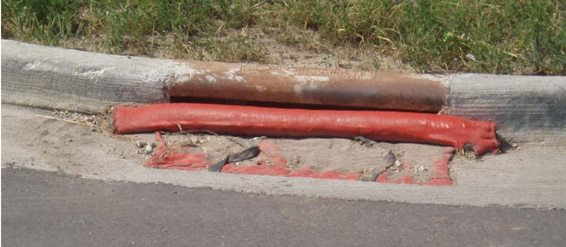
Figure 3.16. Inlet sediment control (Source: Department of Civil, Construction, and Environmental Engineering, Iowa State University)
