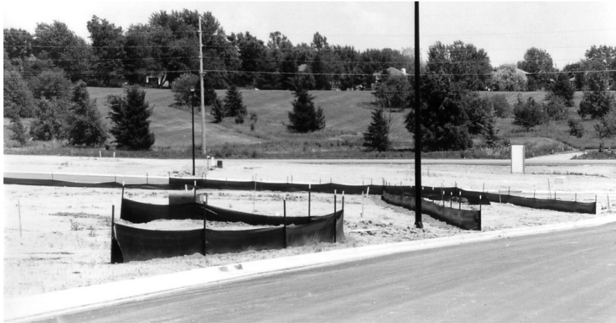
Figure 3.29. Silt fence sediment barrier (Source: Department of Civil, Construction, and Environmental Engineering, Iowa State University)
