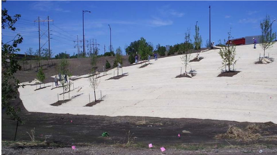
Figure 2.25. Backslope protection (Source: Department of Civil, Construction, and Environmental Engineering, Iowa State University)
