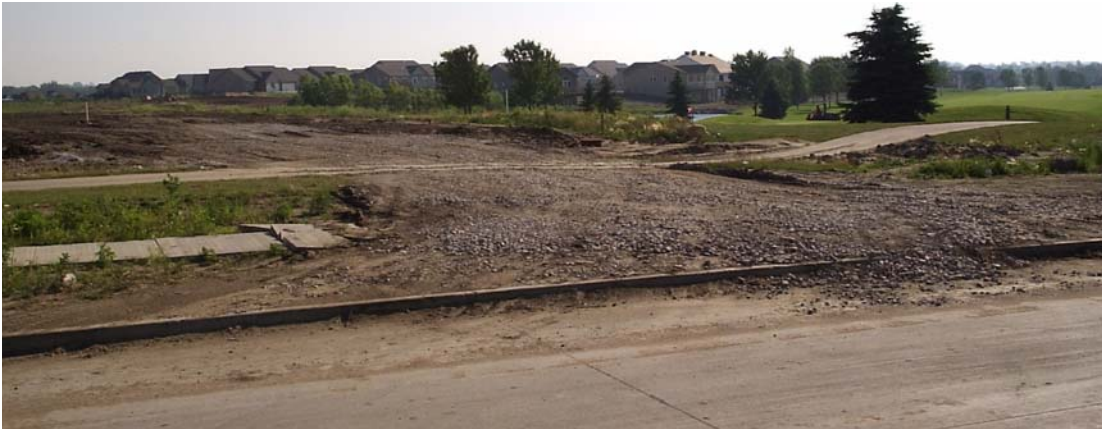
Figure 3.26. Temporary stabilized construction entrance to construction site (Source: Department of Civil, Construction, and Environmental Engineering, Iowa State University)
