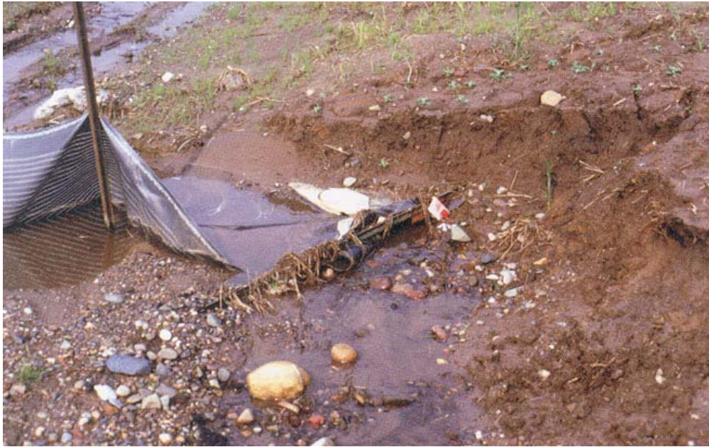
Figure 2.13. Improper silt fence installation (Source: Minnesota DOT)
