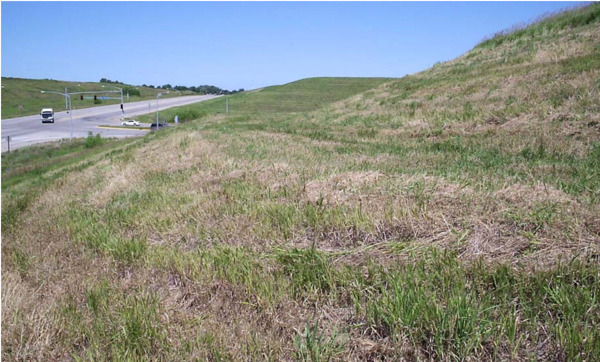
Figure 3.2. Bench cut, profile view (Source: Department of Civil, Construction, and Environmental Engineering, Iowa State University)
