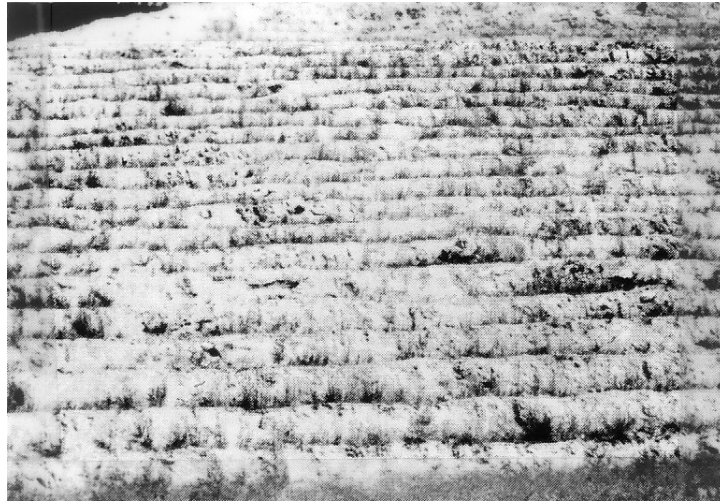
Figure 4.3. Serrated cut (Source: Department of Civil, Construction, and Environmental Engineering, Iowa State University)
