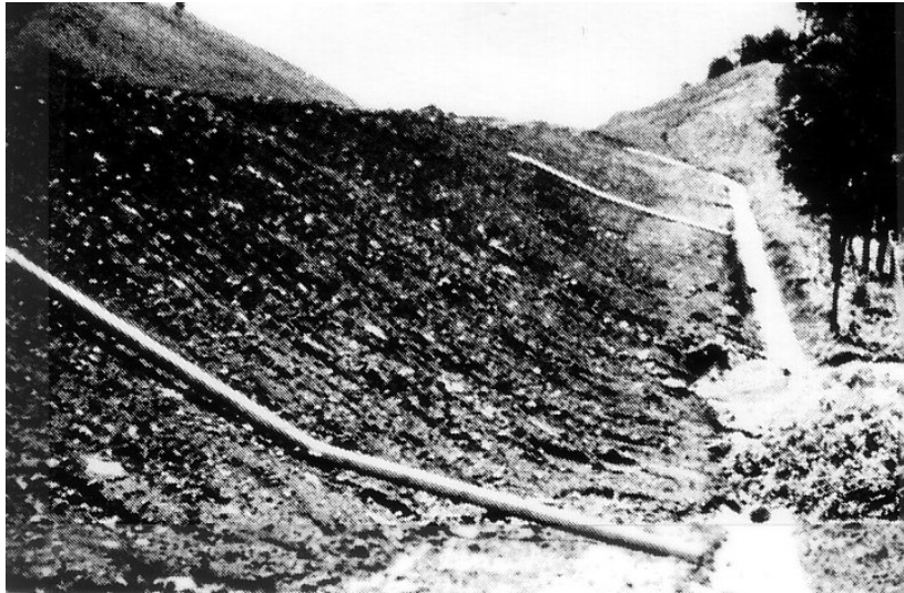
Figure 3.9. Temporary slope drain (Source: Department of Civil, Construction, and Environmental Engineering, Iowa State University)
