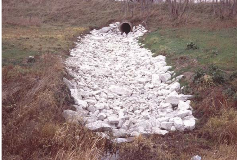
Figure 3.10. Energy dissipator (Source: Iowa DOT)
